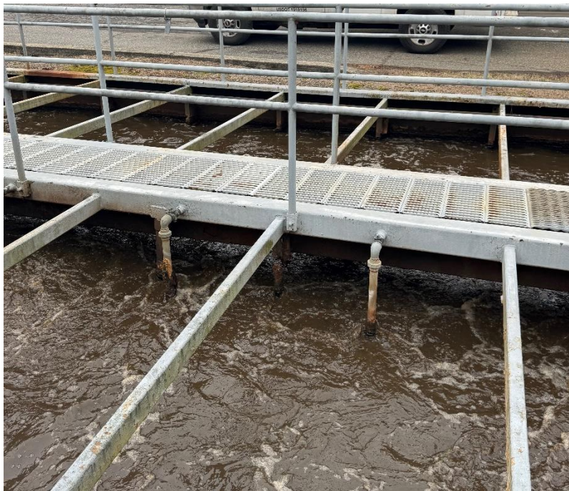
Photo No. 7: Existing Steel Process Tank (Structural Support Deteriorating)
