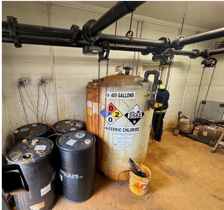
Photo No. 11: Ferric Chloride Chemical Storage
