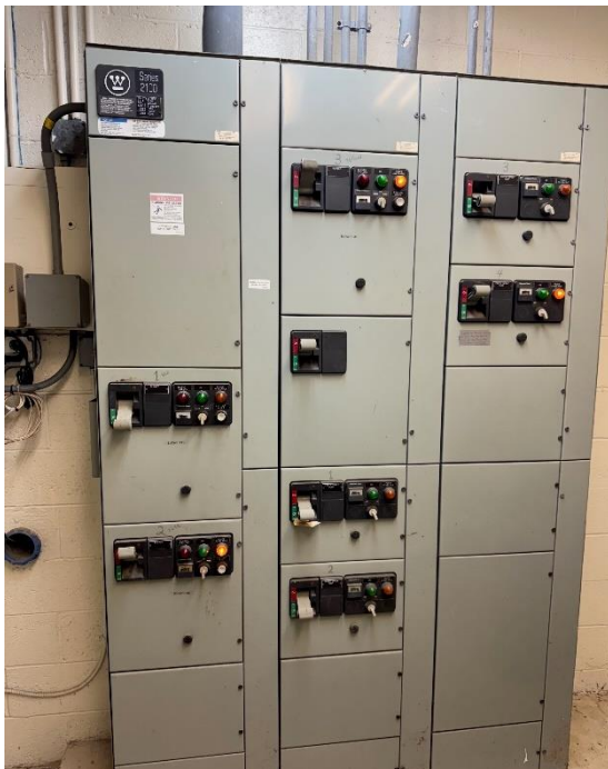
Photo No. 13: Existing MCC
