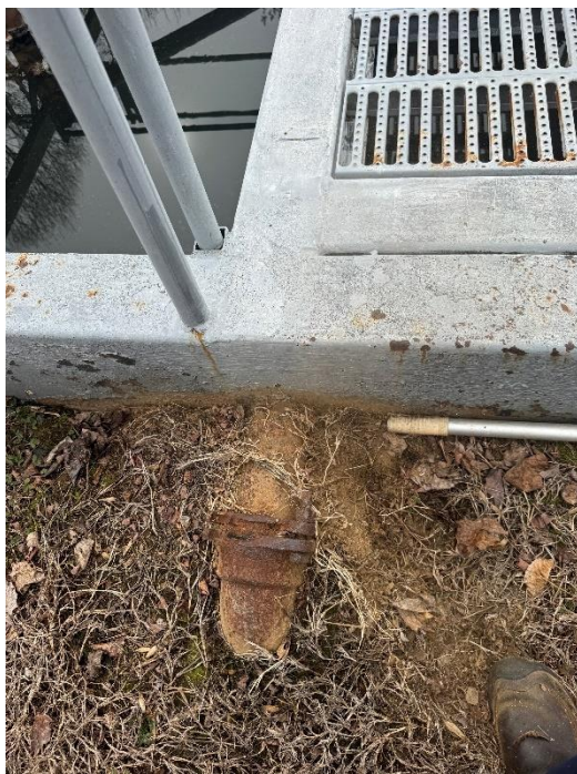
Photo No. 18: Aeration Pipe with Apparent Leak
