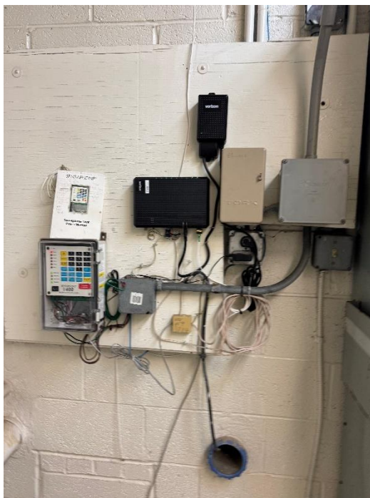
Photo No. 14: Existing Communications/ Wiring
