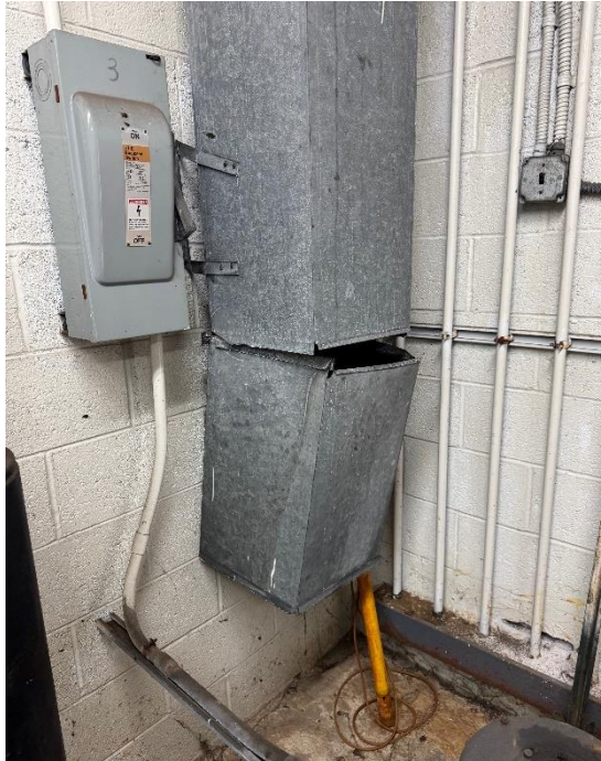
Photo No. 15: Existing Ventilation
