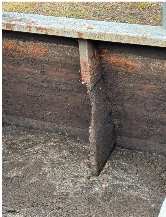
Photo No. 3: Signs of Corrosion/ Deterioration in Steel Process Tanks
